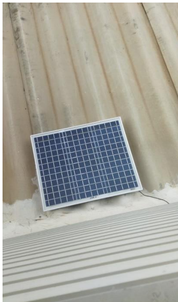
Figura 31. Panel solar instalado
